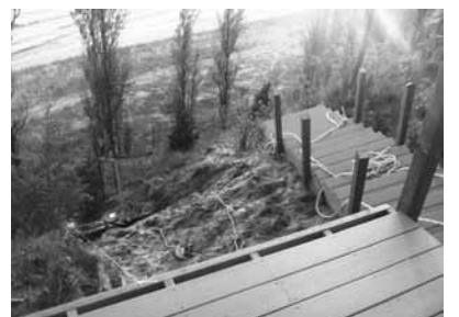
Progress on the Grace Rd. stairway , June 19. PHOTO BY GRACE BANKSTON WILLIAMS
